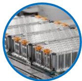
Battery and Energy Storage
